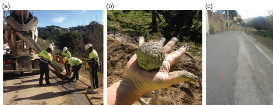
FIGURE 10. (a) Pouring of the concrete, (b) consistency verification and (c) finished trench.
