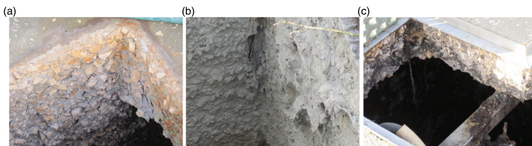
FIGURE 1. Aspects of concrete degradation. Waste treatment unit. Aveiro, Portugal.
