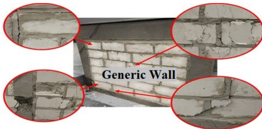
FIGURE 12. Details of cracks and cracks in walls after testing.
