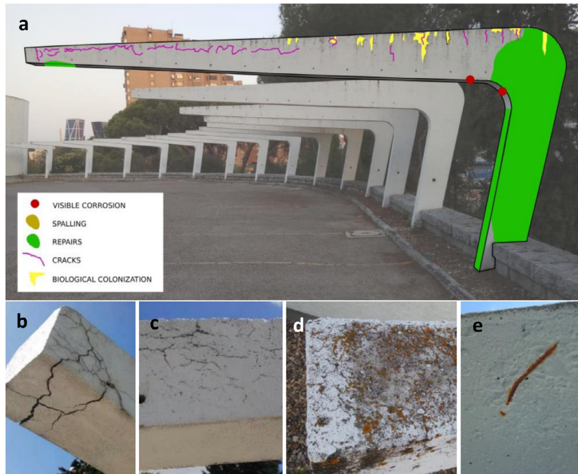
FIGURE 3. Damage mapping in the car park pergola: (a) Diagnosis. (b) Significant cracking. (c) profuse cracking. (d) Biological colonisation. (e) Steel corrosion.
