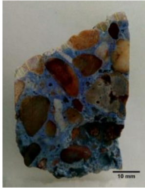
FIGURE 12. Surface of freshly broken core sample drawn from rib-like shell after spraying with thymolphthalein (blue dye = non-carbonated material)
