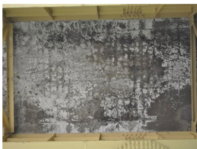
FIGURE 1: The bottom surface of the floor slab with lattice-like cracks (No. 1).
