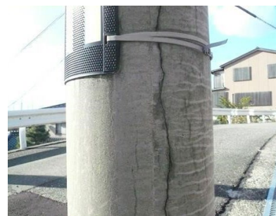
FIGURE 3: Vertical cracks in the PC pole (No. 3).
