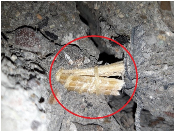
FIGURE 18. Rupture of GFRP rebar in concrete beam after loading.
