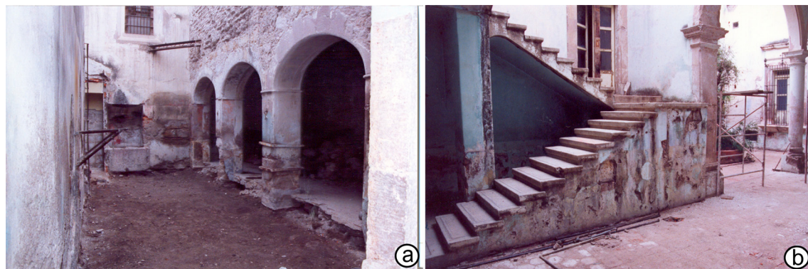
FIGURE 1. Images obtained from the interior of the Casa Terán in 1991. Humidity problems are observed in the lower part of the walls, inferior stairs and structural elements. a) Stable area, currently a covered patio with a cinema area. b) Stairs over the corridor on one side of patio 2.
