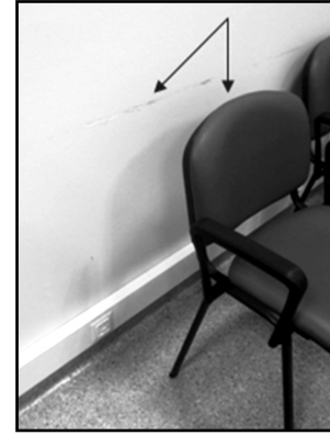
Figure 4. Damaged wall due to the frequent impact of chairs (20).
