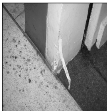
Figure 2. Degradation of tape in a convex corner (20).
