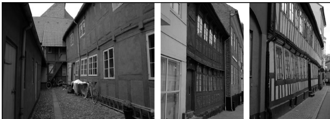
Figure 20. Deformation of structural wood elements due to excessive loading (27).
